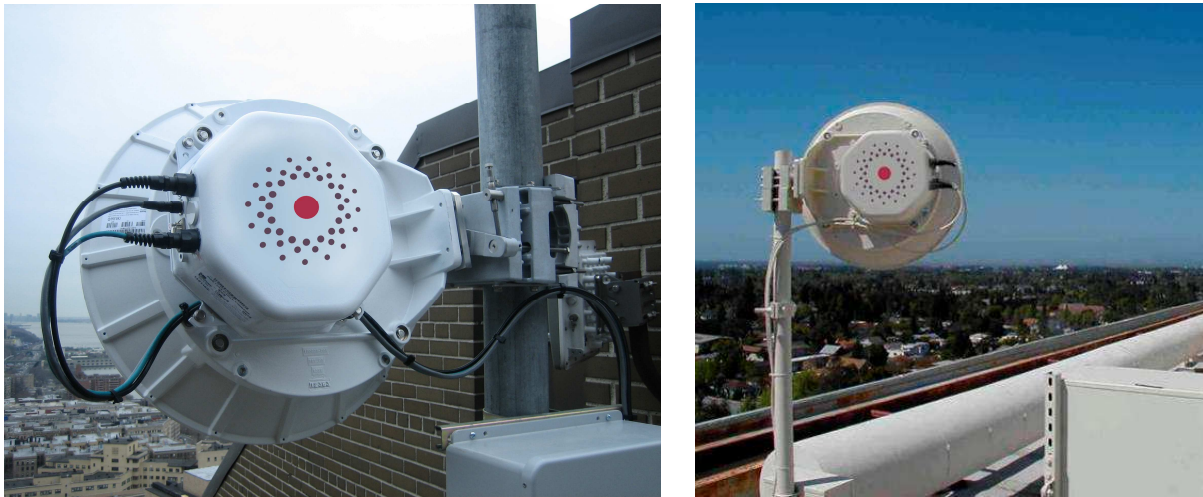
Figure 2: Photographs of a 1.0 Gbps 70/80 GHz radio with a 2ft antenna in typical installations. (Photographs courtesy of GigaBeam Corp.)
